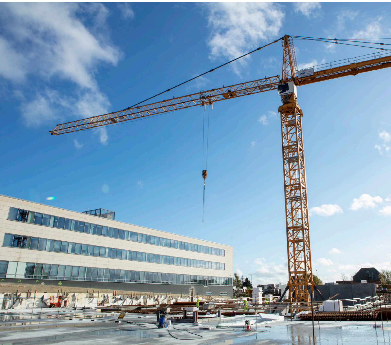
Expansion of JYSK's and Lars Larsen Group's international Head Office. When the two new buildings are finished in April 2022, the JYSK's and Lars Larsen Group's Head Office offers 21,200 square meters for the employees including 200 offices with room for 800 employees, 67 meeting rooms and a brand new auditorium seating 400.
