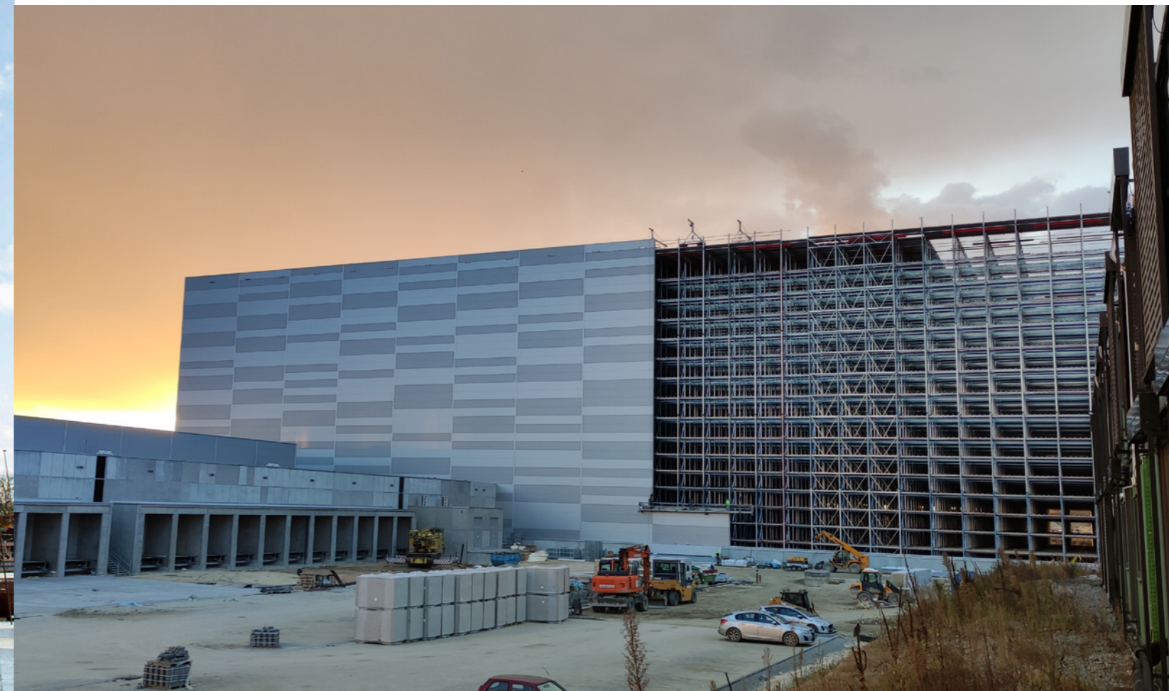
In Ecsér, Hungary, JYSK is building a brand new distribution centre which will serve stores and customers in Hungary, Czech Republic, Slovakia, Slovenia, Croatia, Bosnia and Serbia.
