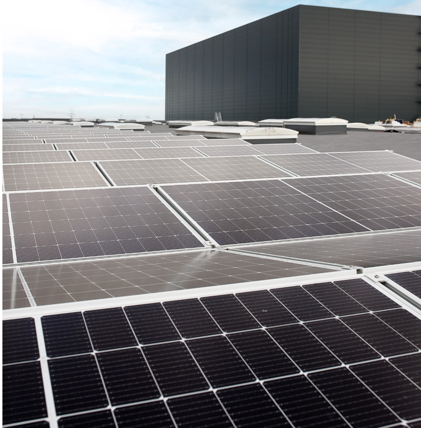
Solar panels make the Vision Park warehouse self-sufficient in energy supply.
